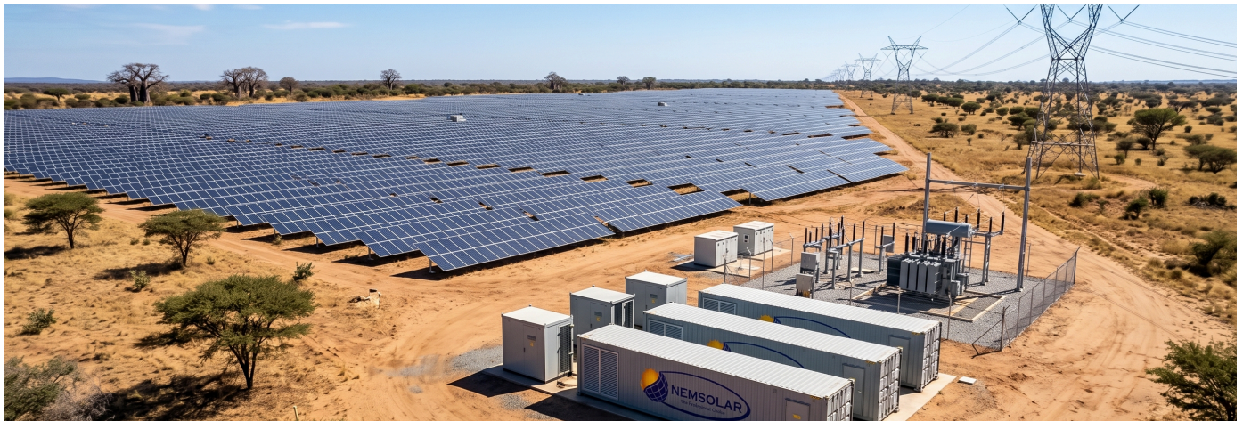
Grid-connected solar with battery storage and transmission infrastructure.
