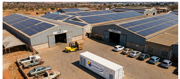
Processing plant with rooftop solar & BESS — Lusaka, Zambia.
